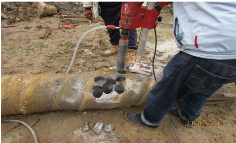
Fig. 3. Coring concrete samples of the uplifted RIT pile ( L = 6 m, D = 0.4 m, Essalema City, Tunis)
