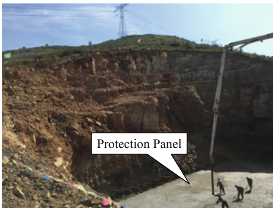
Fig. 8. Construction of the UHV tower foundation on mountains; Protection panel was being pouring
