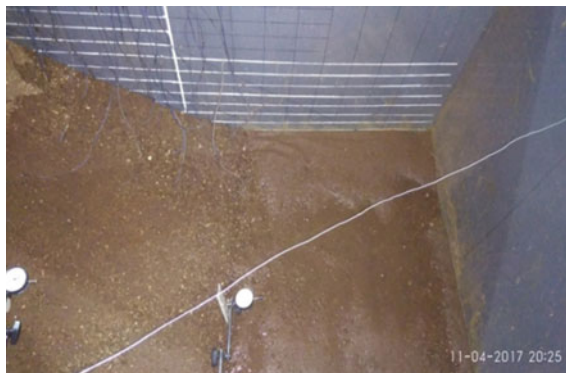
Fig. 13. Slope failure -28° [soil - 1]
