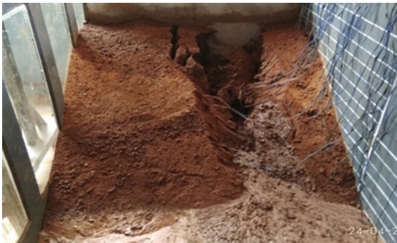
Fig. 23. Slope failure - 30° [soil - 2]
