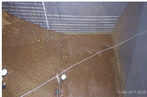
Fig. 13. Slope failure -28° [soil - 1]
