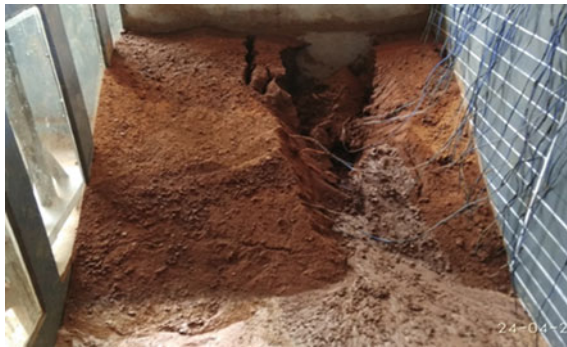
Fig. 23. Slope failure - 30° [soil - 2]
