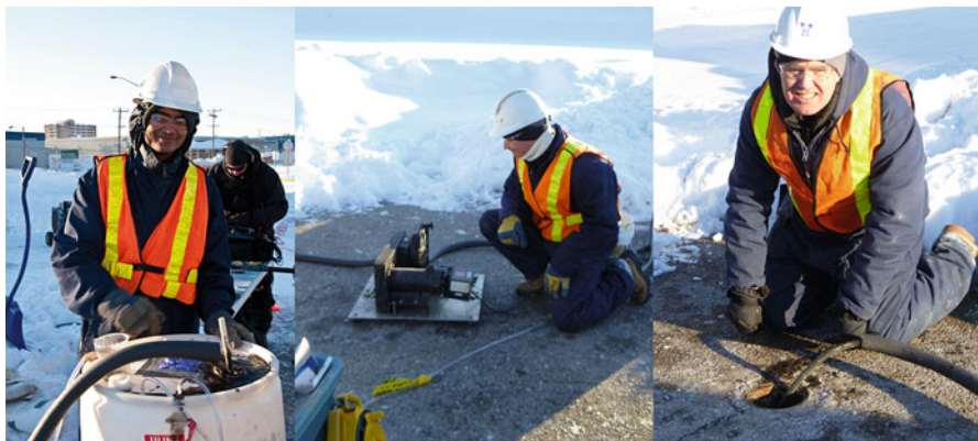
Fig. 7.6 Photos of a constant head injection showing the reservoir (left), pump (center), and flush-mount wellhead (right)
