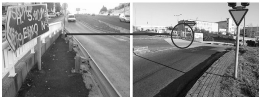
Fig. 10.2 Inadequate pedestrian infrastructures. Source: Photos by the author
