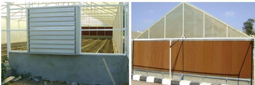
Fig. 16 Fan and pad cooling system. ( Left ) Exhaust fan located on the leeward side of the greenhouse, ( right ) cross fluted cellulose pads placed vertically in the opposite wall of exhaust fans
