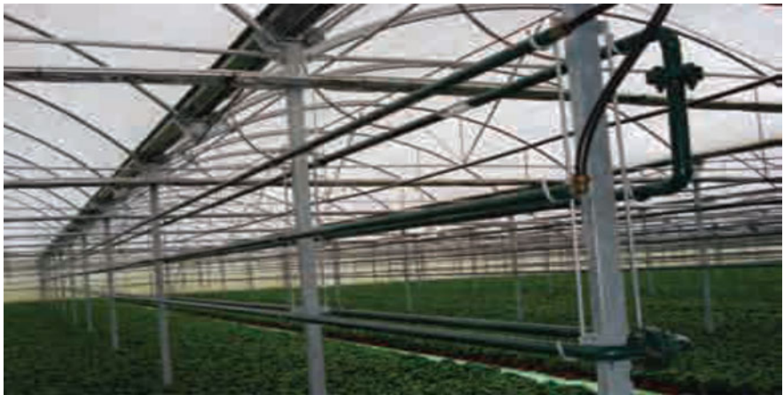
Fig. 8 Heating pipes for dissipating the produced heat
