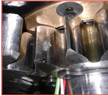
Fig. 2. Pitting located on the test sun
