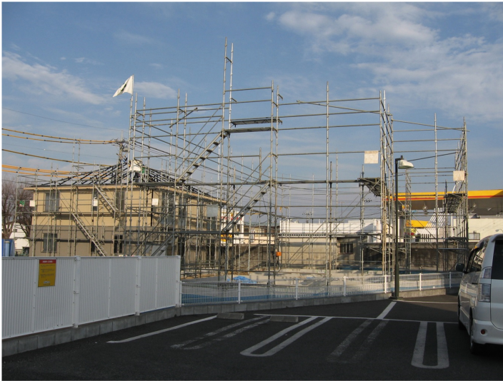
Fig. 3. Scaffolds erected using the Methods to Erect Scaffolds First for low-rise construction.
