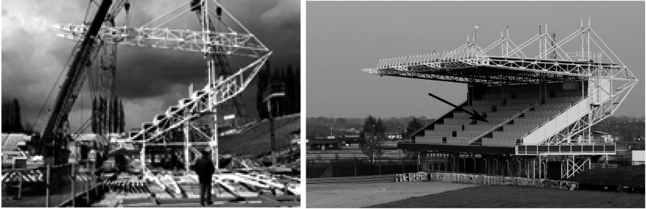
Fig. 1. Portable, temporary grandstand for media with latitudinal vomitory ; on the left - assembly of steel structure at the Silesian Stadium in Chorzow, Poland; on the right - new location 300 km from the original one (the arrow indicates the vomitory position); (Photos: author)
