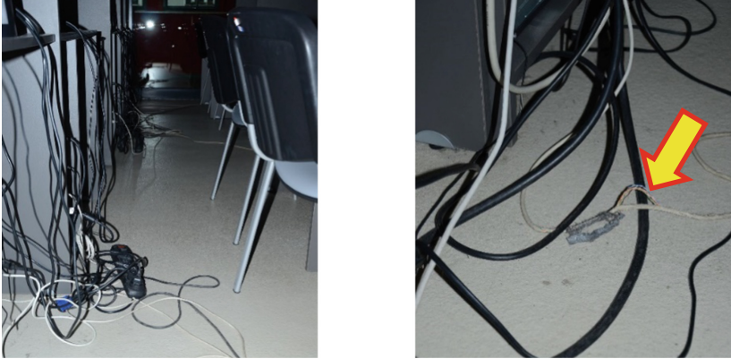
Fig. 4. Distribution of utilities - electricity and network. Dangerous and susceptible to damage. Source: author's archive.
