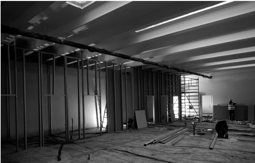
Fig. 3. Photo of the 3D printing factory under construction – skylights in production room, photo by the author.
