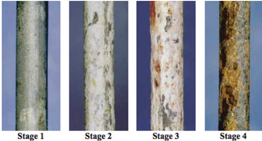
Fig. 4.18 Cable wires subjected to corrosion at different stages, as defined in NCHRP report 534. (Chavel and Leshko 2012)
