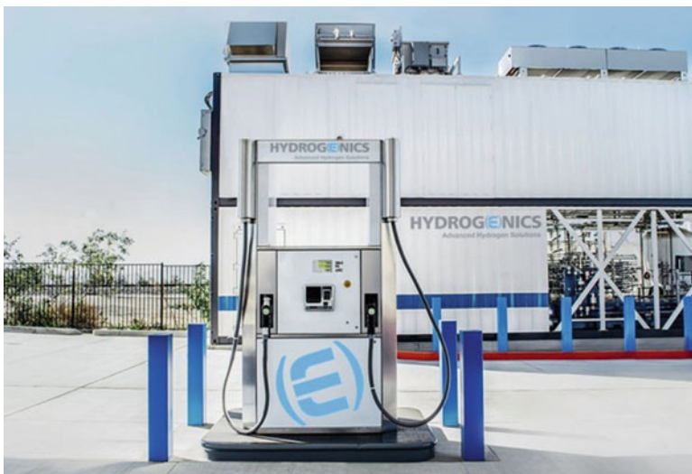
Fig. 2.10 Typical infrastructure of hydrogen filling stations
