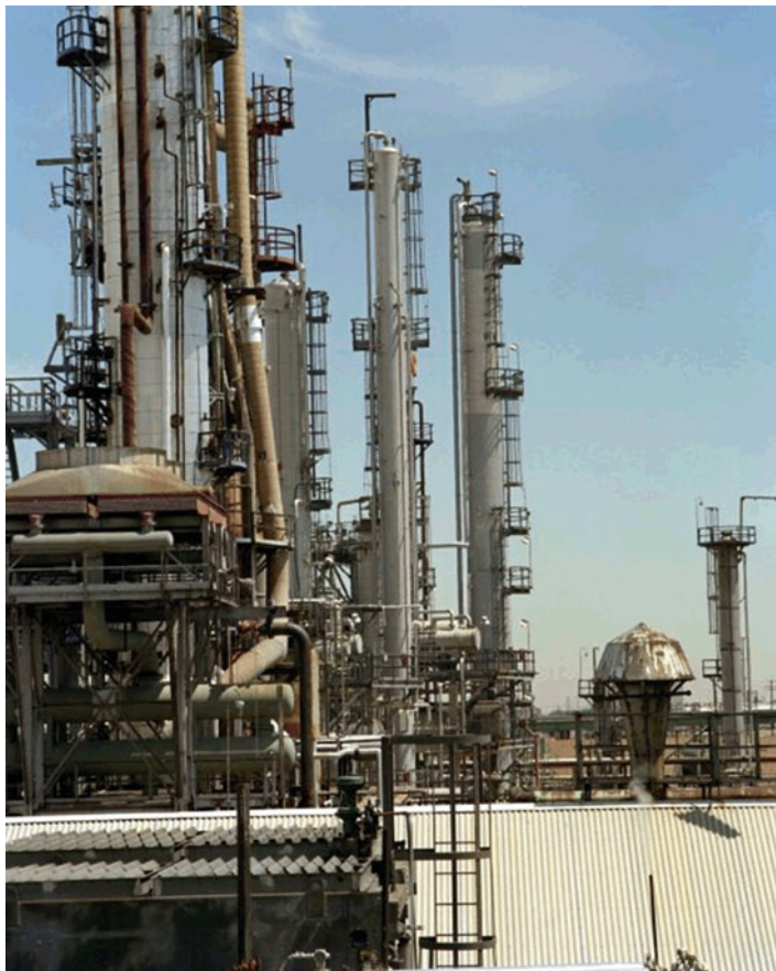
Fig. 1.27 Hydrogen production plant
