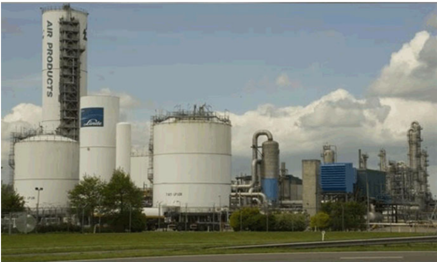
Fig. 4.4 Cryogenic air separation plant with heat exchanger and distillation column towers
