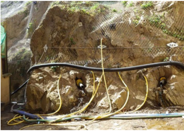
Fig. 14 Containment netting and active drainage installed into a mixed lithology rock mass with compartmentalised groundwater domains
