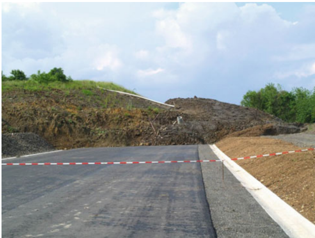
Fig. 7 Landslide toe filled the motorway cut on the first day of sliding. Further movement of approx. 35 m took place over the following three days
