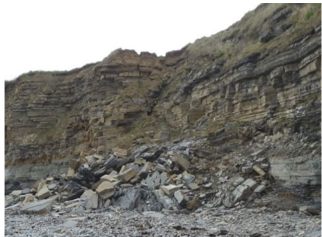
Fig. 9 Compound failure in alternately bedded Jurassic Blue Lias mudstone and limestone strata
