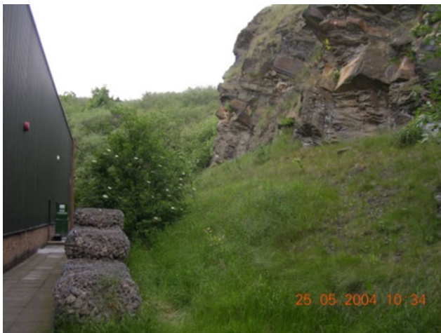
Fig. 10 Undermining of sandstone blocks due to mudstone weathering, with gabion wall protecting building
