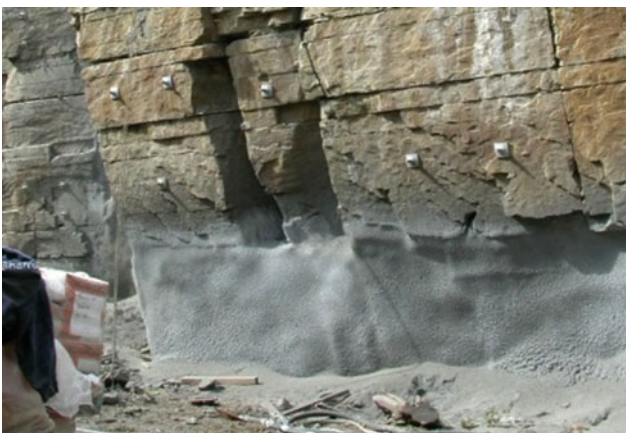
Fig. 15 Cover of exposed mudstone bed preventing air and water access
