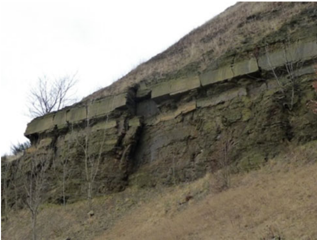
Fig. 6 Mudstone ravelling undermining a sandstone bed. Coal Measures, Sheffield
