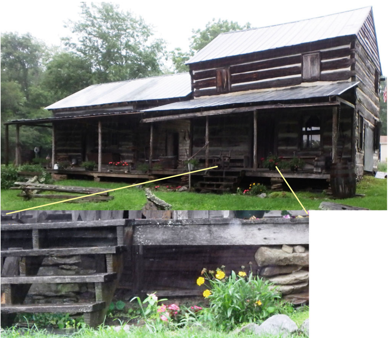
Fig. 1 Photo of an historic building in rural United States with an enlarged inset of the stacked stone columns for the porch and the log foundation in the background (Hempen 2015). Small horizontal vibrations may be damaging to this structure
