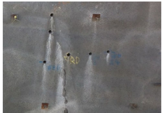
Fig. 12 Inclusion of in slope raking drains to channel water from the limestone bed seen in Fig. 11 and additional weepholes
