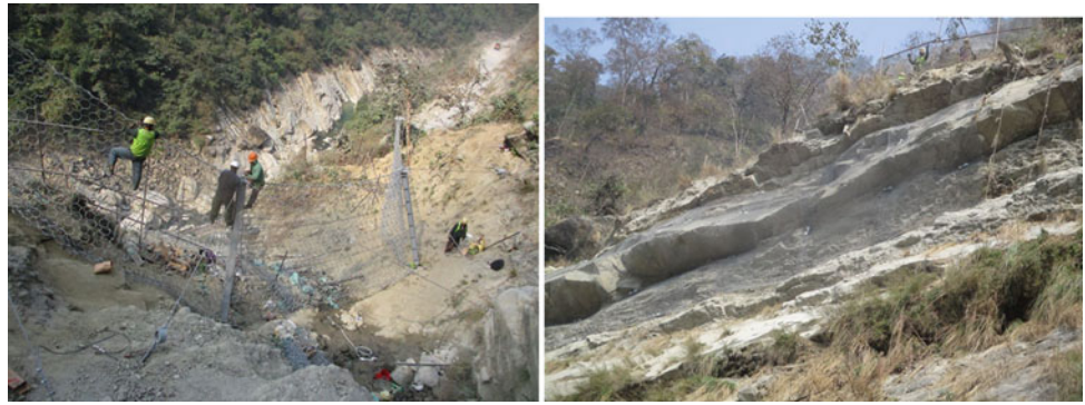
Fig. 4 Model site in Siddhababa. Skilled labors and engineers are installing barriers on left photo and on right photo rock nets installed on hanging sandstone bed
