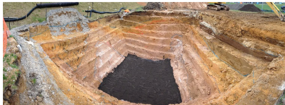
Fig. 7 800 mm thick granular filter layer installed at the base of the excavation
