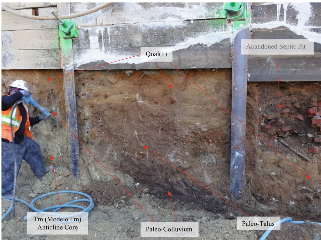
Fig. 7 Excavating the Yucca Project basement bulkhead. See Fig. 6b for a graphic illustration of this exposed section along Argyle Avenue. Photo by Steven Kolthoff
