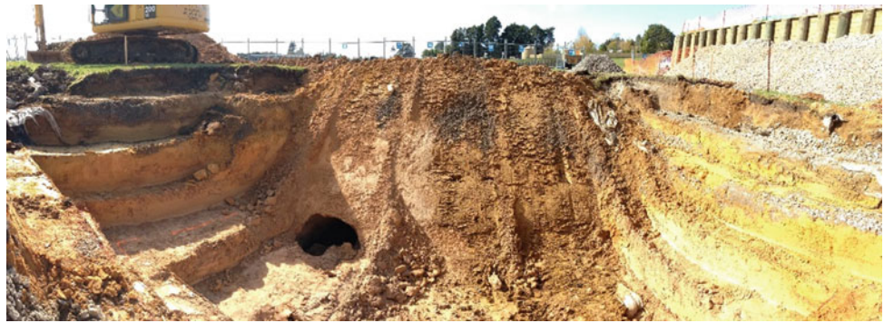
Fig. 6 Approximately 1 m diameter cavity observed during construction
