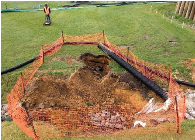
Fig. 4 Sinkhole observed in the playfield of the school. GPR survey underway
