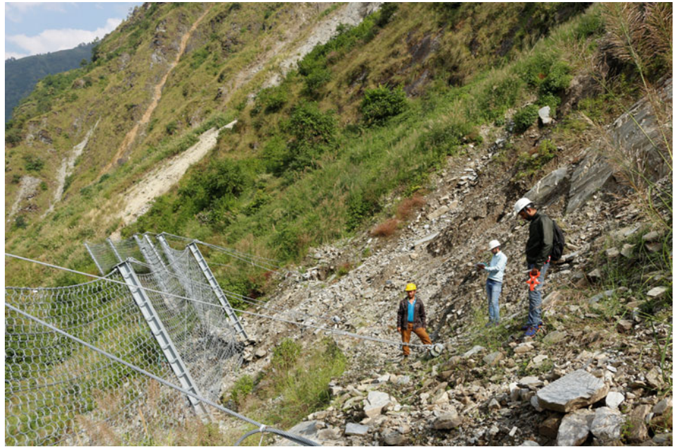
Fig. 6 Already installed rockfall protection barrier on uphill slope of Upper Bhotekoshi Hydropower Project
