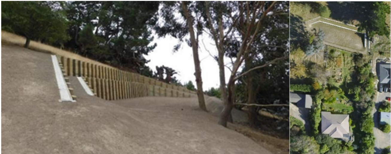
Fig. 5 Terrace and berm RPS on Avoca Valley Road. The image on the right is a Google Earth image of property and terrace upslope
