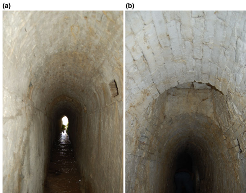
Fig. 5 a The drainage system: branch A. b Vertical shaft in the branch A
