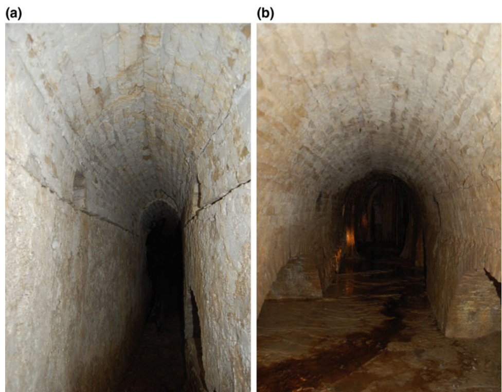
Fig. 6 a The drainage system: branch B. b Vertical shaft in the branch B
