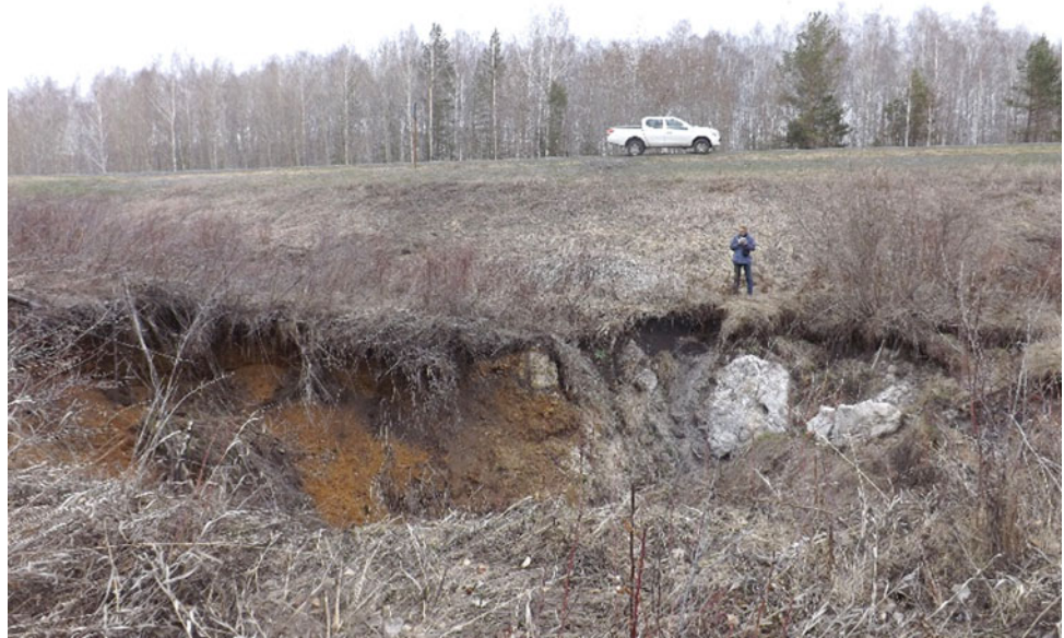
Fig. 4 Karst-suffusion failure on the 8th kilometer of the road Bogdanovich—Sukhoy Log
