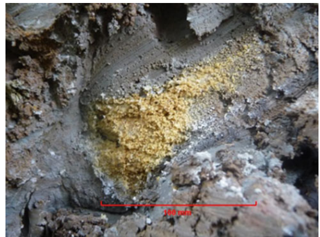
Fig. 12 Saccharoidal selenite with hydrous iron oxide surface staining in weathered Lower Lias Clay
