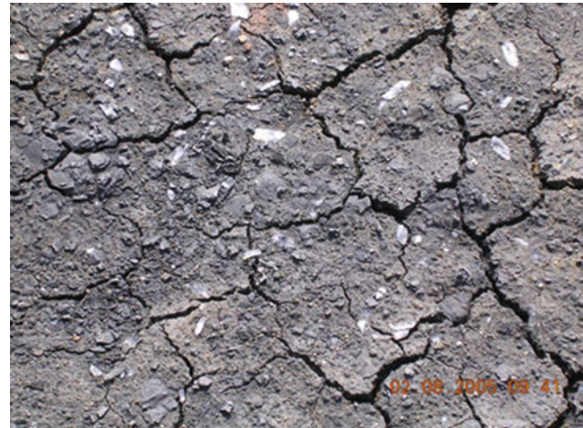
Fig. 6 Rapid deterioration due to pyrite oxidation of highway formation surface showing desiccation and selenite
