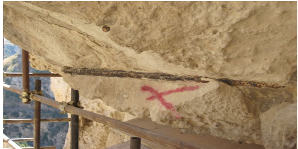
Fig. 12 Failure of reinforcement with steel elements
