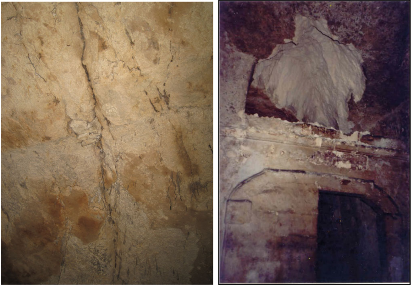
Fig. 8 Fracture example and collapse due to fracture in Matera “Calcarenite”
