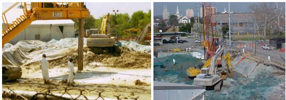
Fig. 3 Right photo: Crane-mounted auger ISS, Left photo: Note change in grade for ISS beginning at water table
