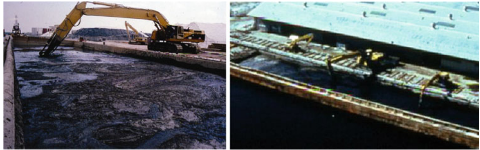
Fig. 4 Right photo: Mixing cement into barge of sediment, Left photo: Port-side treatment
