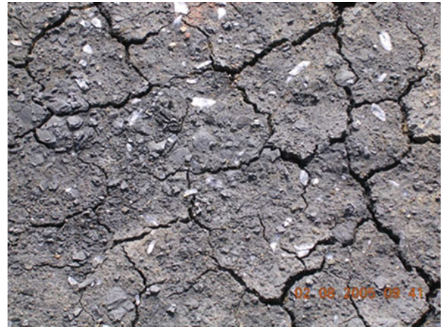
Fig. 6 Rapid deterioration due to pyrite oxidation of highway formation surface showing desiccation and selenite
