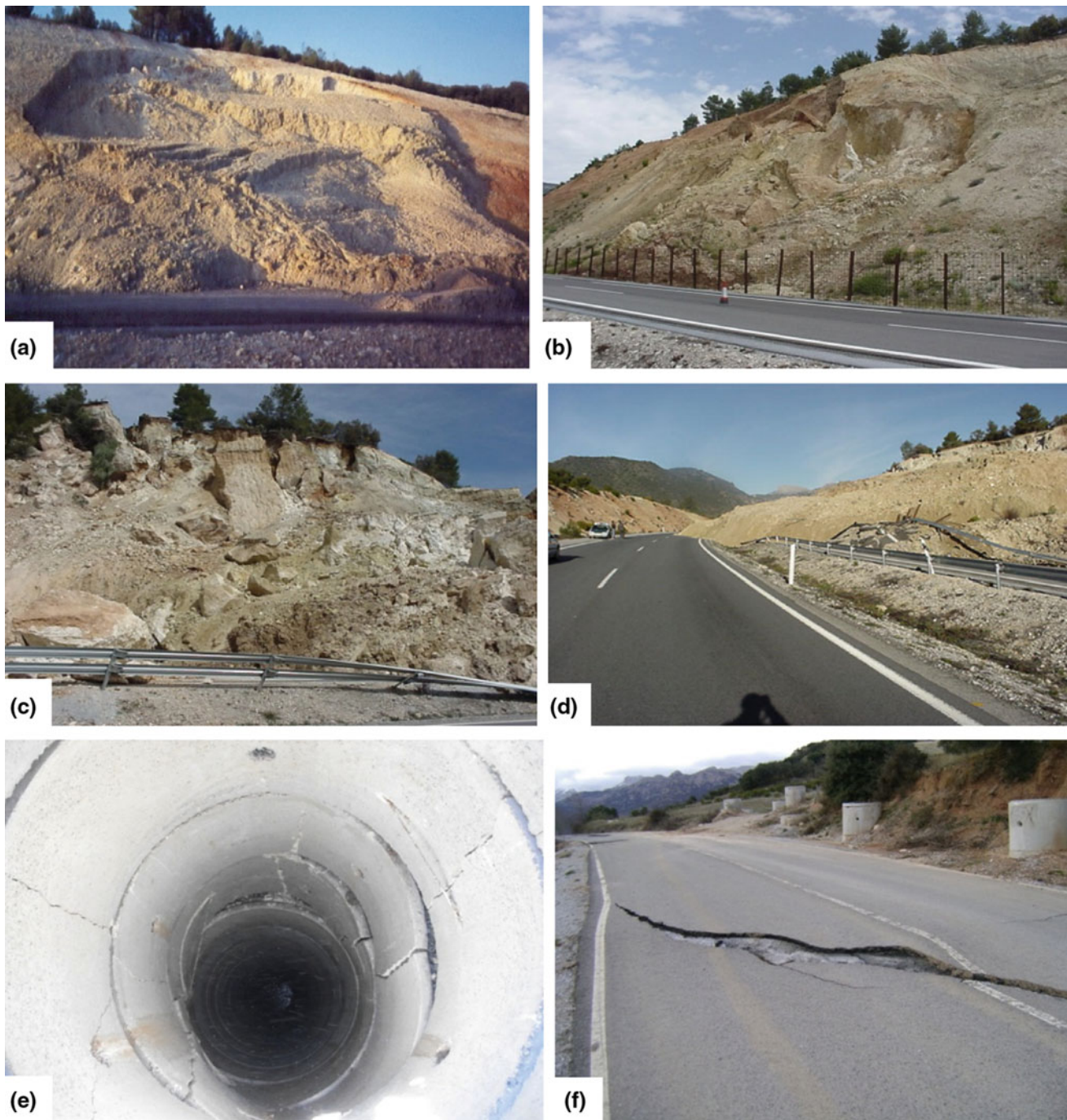
Fig. 2 Damages: a landslide (October 1991), b landslide (May 2000), c, d main landslide (March 2001), e broken drainage well (May 2006), f crack near the landslide crown (November 2009)
