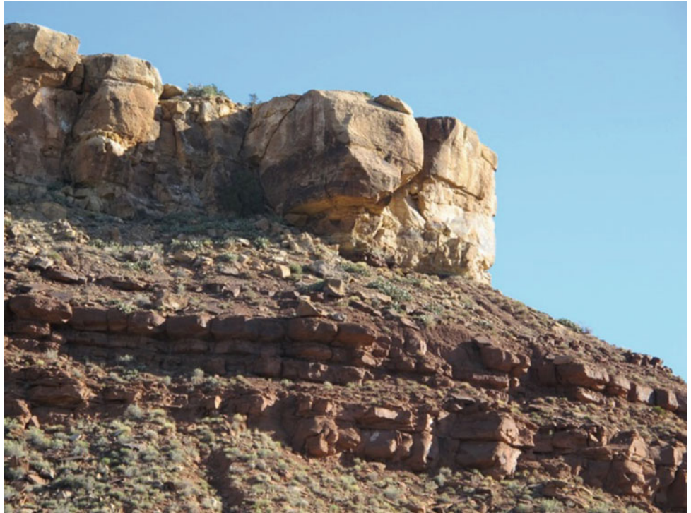
Fig. 6 Undercutting of the Shinarump Conglomerate Member by the Moenkopi Formation between Site 3 and Site 4, resulting in potentially unstable blocks of the Shinarump Conglomerate Member
