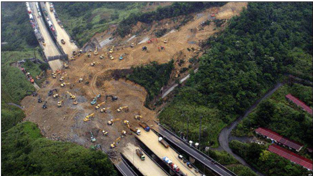
Fig. 1 Landslide after rain in 2010, Taiwan
