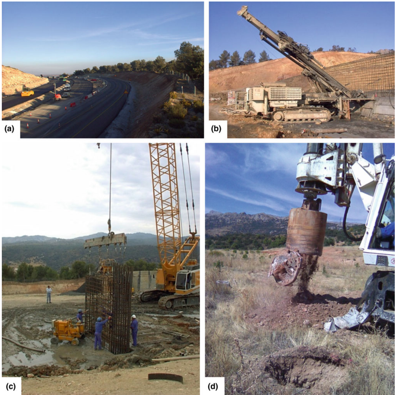
Fig. 3 Countermeasures: a provisional roadway (April 2001) b anchors (October 2001) c retaining barrier (August 2001) d drilling new wells (October 2009)
