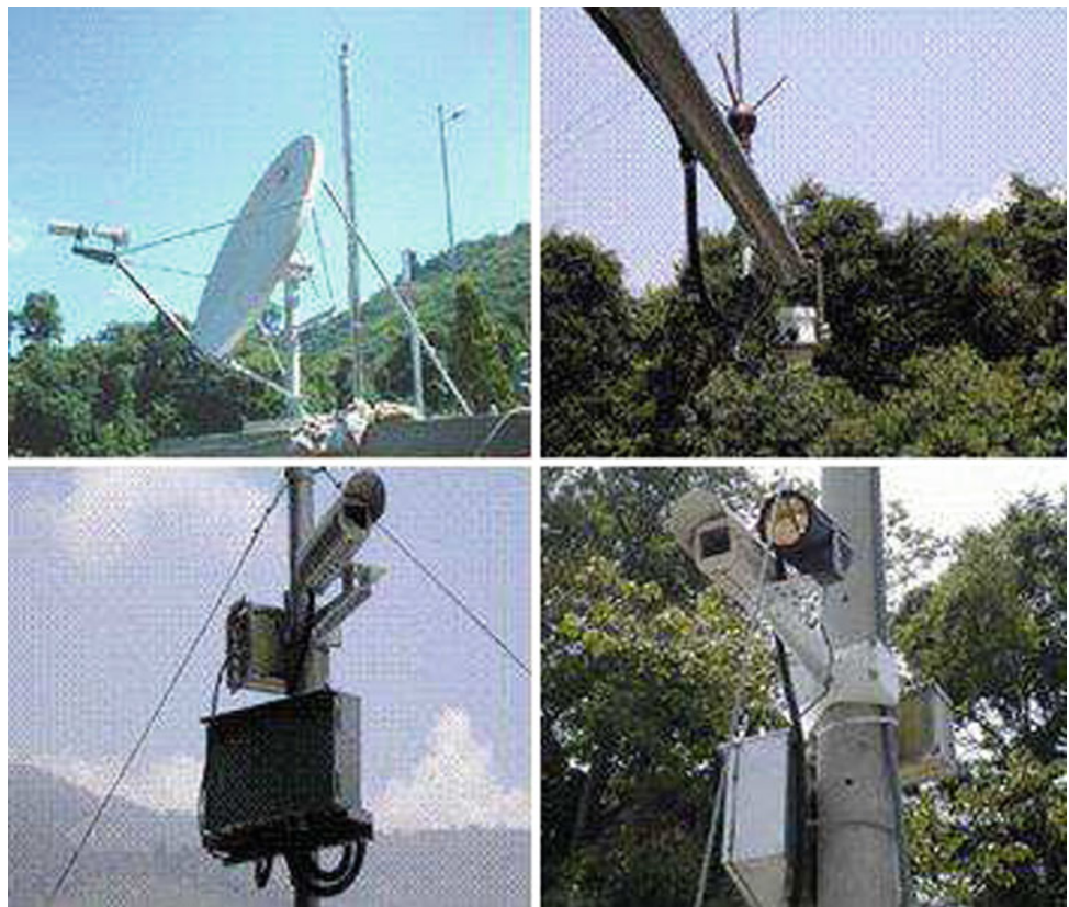
Fig. 4 The equipment at the Fengqiu Debris flow monitoring station include 1 rain gauge, 2 CCD cameras, 2 geophones, 4 wire sensors and 1 water level meter
