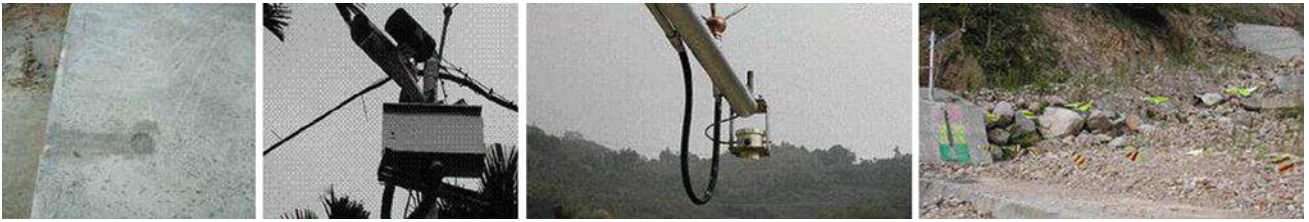
Fig. 5 The equipment at the Shang'an debris flow monitoring station includes 1 rain gauge, 1 CCD camera, 1 geophone, 2 wire sensors and 1 water level meter
