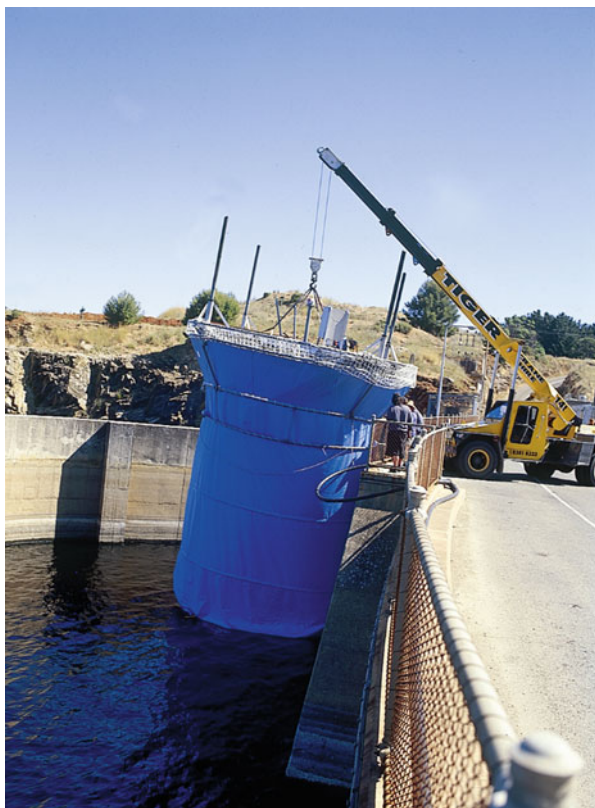
Fig. 6.4 A surface mounted mixer being deployed in Myponga Reservoir in South Australia
