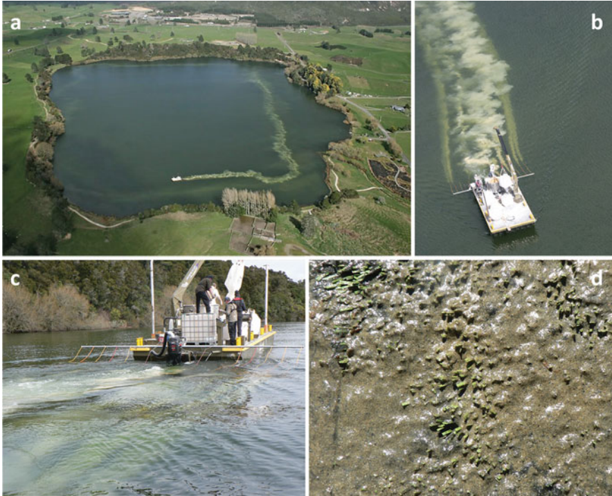
Fig. 7.16 (a–c) Applying <0.5 mm Aqual-P ® as a sub-surface slurry injection from a barge. (d) Aqual-P ® coverage of an artificial turf substrate used to check the evenness and thickness of the Aqual-P ® cover across the lake bed [photos a and b by Andy Bruere, BOPRC; photos c and d by M. Gibbs, NIWA]
