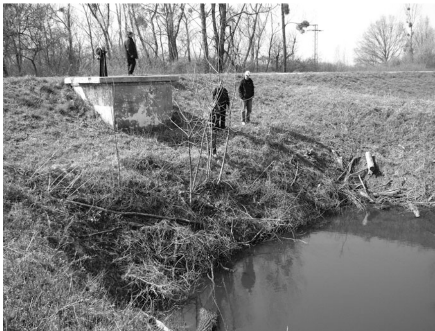
Fig. 2 The outlet structure of the protection dam on the left-hand side of the Latorica River
