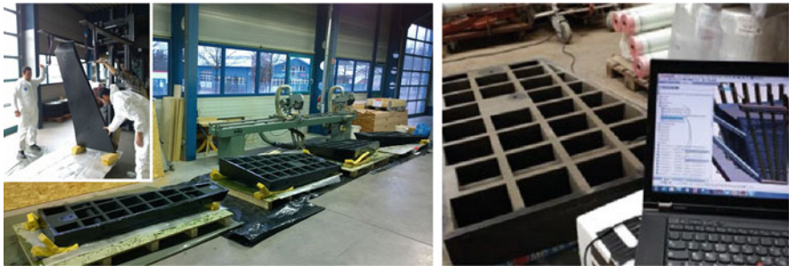
Fig. 26.21 Manual application of epoxy resin on the surfaces of the 3D-printed formwork elements. (© Ed. Züblin AG, reprinted with permission)
