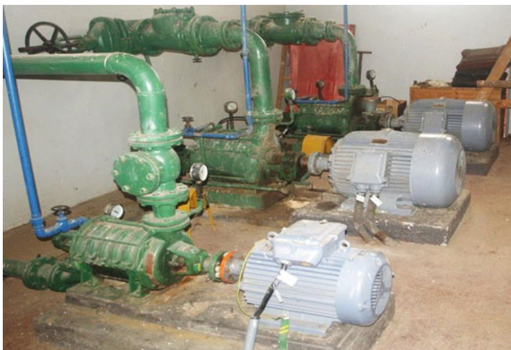
Fig. 3 Small irrigation pumping station for 300 ha (Photo: Jurík, 2016)
