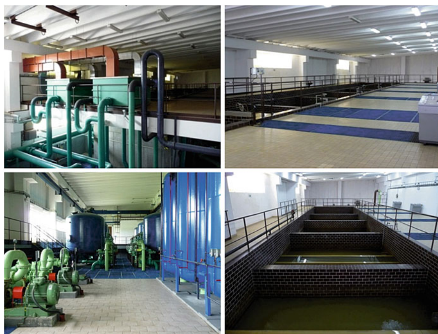
Fig. 13 WTP Kúty (aeration units, pump and filtration halls)
