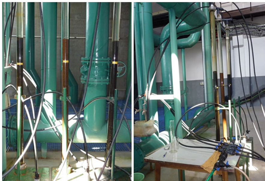
Fig. 15 Filtration equipment – filtration columns
