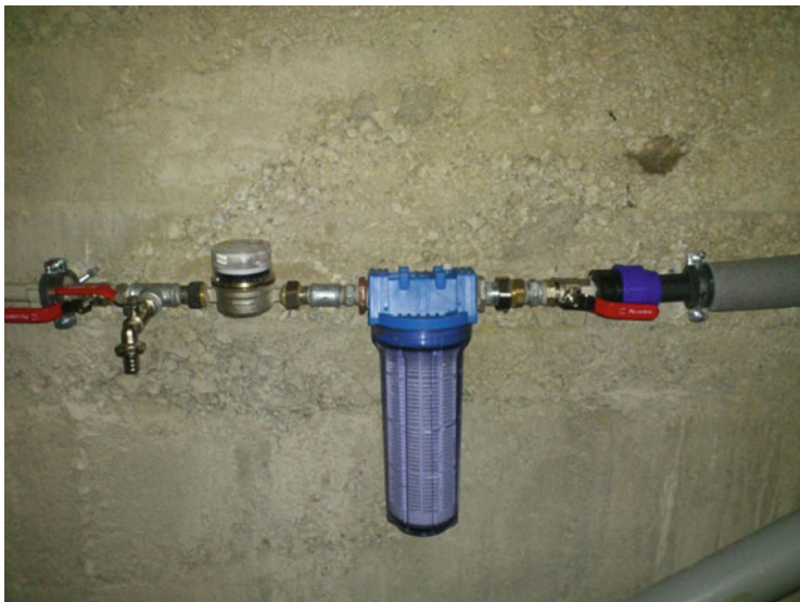
Fig. 4 Connecting pipes, filter, and water meter
