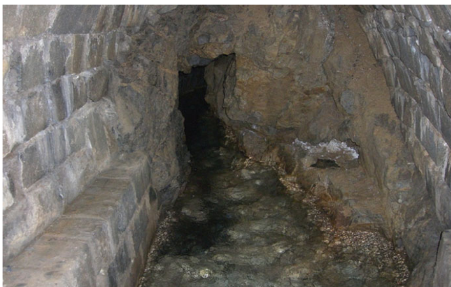
Fig. 15 The view into the side chamber with the groundwater flow from the rock massif (Photo: M. Fendeková)
