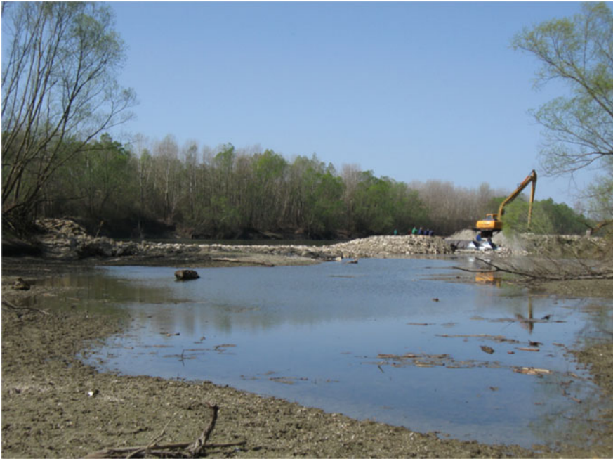
Fig. 20.6 The partially demolished stone closure of the Drávatamási Upper side channel (photo by Tibor Parrag)
