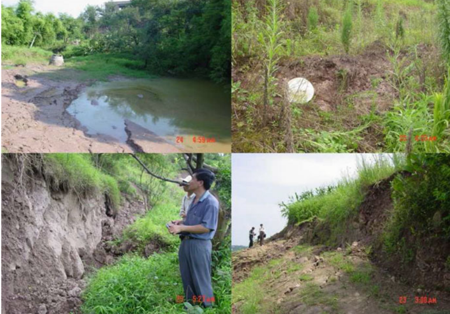
Fig. 3.8 Penetration at the trailing edge of the landslide (the upper-left figure), crack at the trailing edge of the landslide (the upper-right figure), the steep surface between the failed body and the terrain (the lower-left figure), and road deformation in the front edge of the landslide (the lower-right figure)
