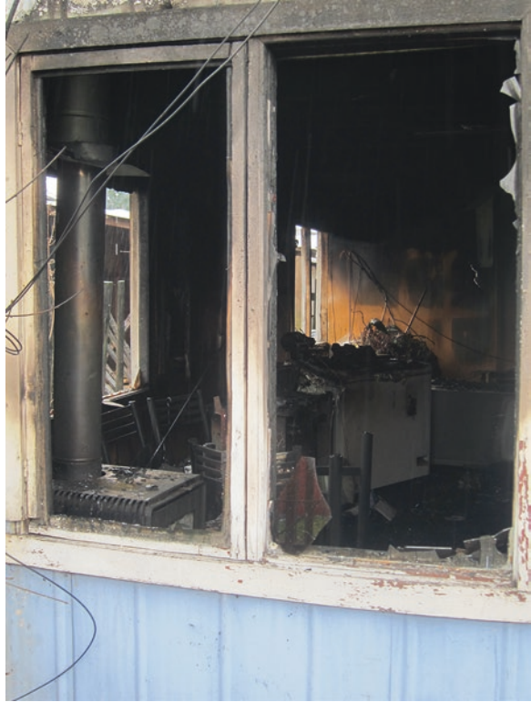
Image 6.3 Interior of a home in Puerto Aysén destroyed by fire in 2015. (Photo credit: Eric Harrison Thomas)
