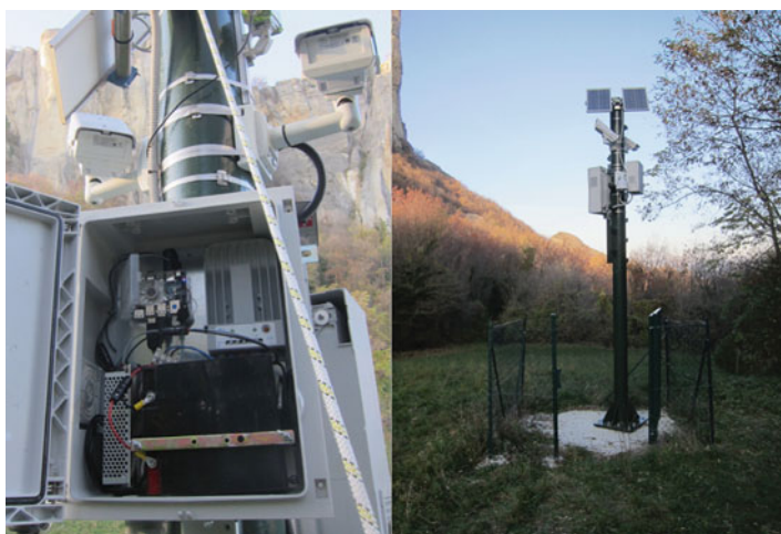
Fig. 13.1 Left: Beesper SmartBridge prototype. Right: Beesper SmartBridge prototype installed on a pole
