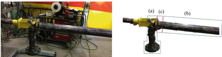
Fig. 4. Illustration of REF, ADD and connection point on a pipe spool assembly in a fabrication facility. On the left, a photo from a fabrication shop representing an assembly ready for welding. On the right, this assembly is analyzed for the purpose of the methodology. (a) Reference consists of a flange, a pipe, and an elbow. (b) Addition is a straight pipe. (c) The weld point shared between REF and ADD.
