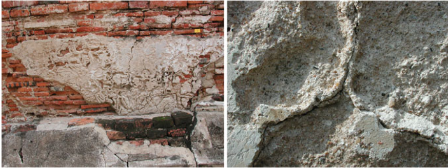
Fig. 7 Alveolar weathering of renders on the enclosure wall (MHT 1, left, and detail from MHT 6, right). As can be seen on the right, the ridges are often preserved along cracks
