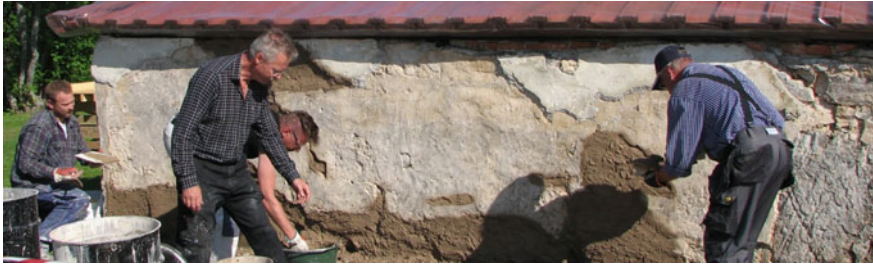
Fig. 3 Mortars are applied with a trowel onto the wall. Old mortars can be distinguished by color and texture, here as the white and yellowish surfaces in the picture
