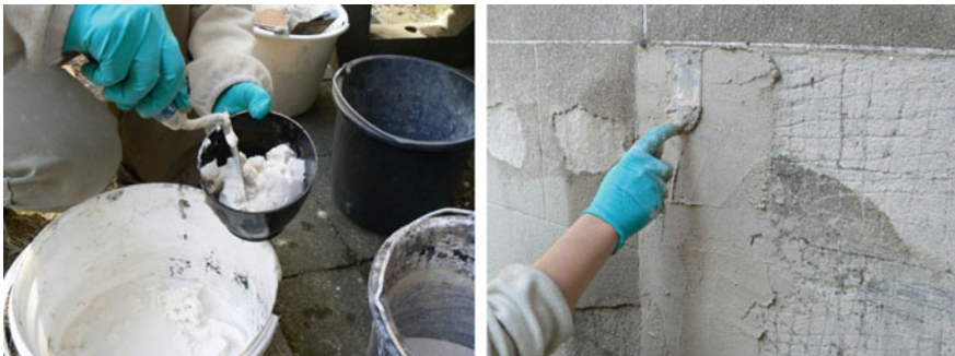
Fig. 8 Final stage to repair damaged exterior stone imitations. The stone imitation render is refabricated and spread onto the façade (Govaerts 2012)
