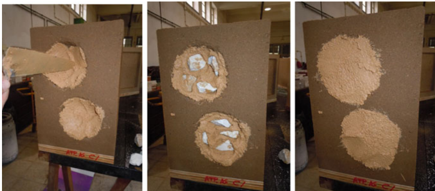
Fig. 4 Application of the mortar MRE on a standard deep voids defect of the Av rammed earth
