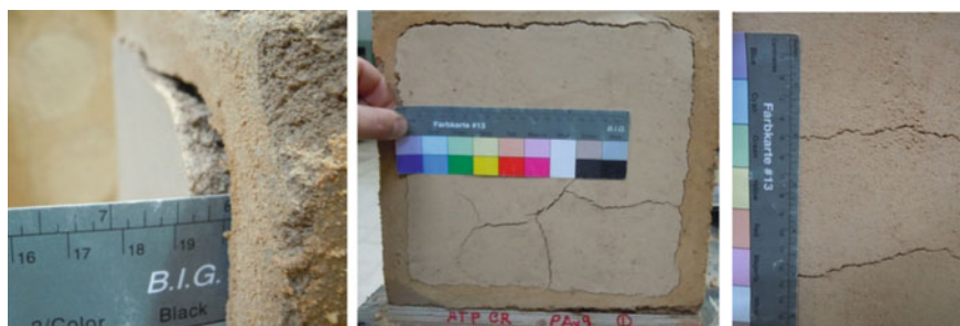
Fig. 5 Mortar MRE_NC15 applied in block BAv on standard superficial defect: left, detachment of the mortar; center, cracks; and right, detail of large cracks
