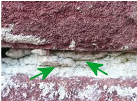
Fig. 1 Horizontal layering (see arrows) in an uncarbonated air lime repointing as a result of freeze-thaw cycling
