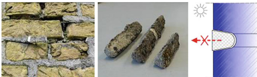
Fig. 4 Detachment of repointing caused, in particular, by thermal deformation enhanced by a wrong cross-sectional form (V-shape instead of rectangular) of the repointing
