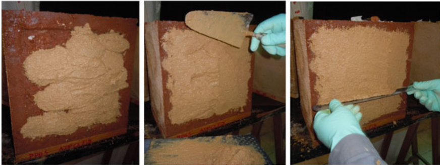
Fig. 3 Application of the mortar MRE_CL15 on a standard superficial defect of the PD rammed earth
