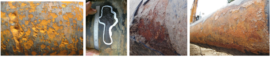
Fig. 1. Example of different corrosion shapes and surfaces.
