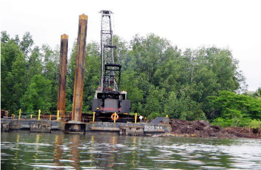
Fig. 13.5 Dredging activity to create pipeline route through the mangrove forest in Bakana town, Niger Delta, Nigeria. (Credit: A.O. Numbere)
