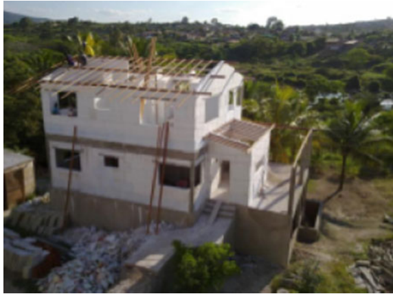
Fig. 23 Examples of building constructions that employ gypsum (gypsum house under construction, Gravató-PE)
