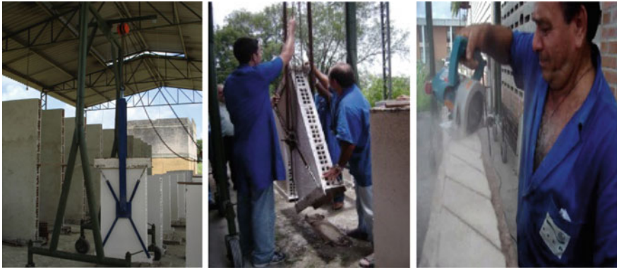
Fig. 6 Details of the handling the specimen and execution of top bottom surface
