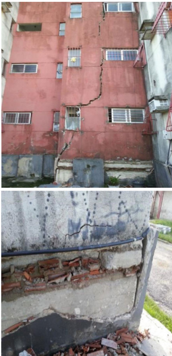
Fig. 1 Examples of pathological manifestations observed, namely, a detail of masonry crushing between foundation beam and ground floor slab
