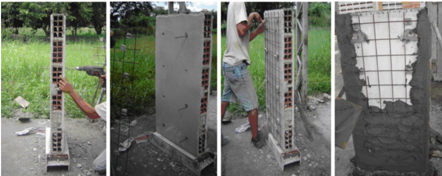
Fig. 5 Steps of drilling, installation of connectors, steel mesh, mortar coating and spacers
