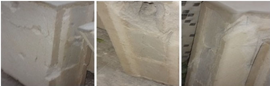
Fig. 15 Rupture of concrete block prisms coated with 3.0 cm of mortar and an additional reinforced mortar layer
