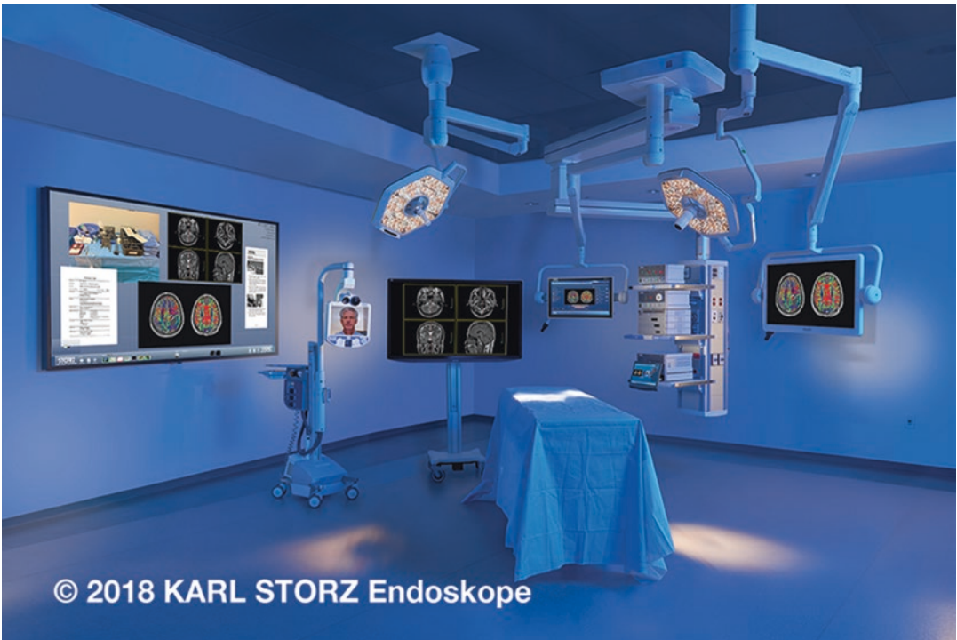
Fig. 4.10 Operating rooms today, such as the ORI ® integrated suite above, must encompass a broad range of systems for data and image management, device control, and more. Each piece of equipment and its functional compo-
