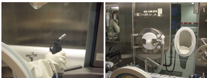
Fig. 21.5 Automated CIP of lyophilizer loading/unloading zone (right) and manual wash-in-place of filling compartment (WIP, left); equipment located at F. Hoffmann-La Roche, Basel, Switzerland
