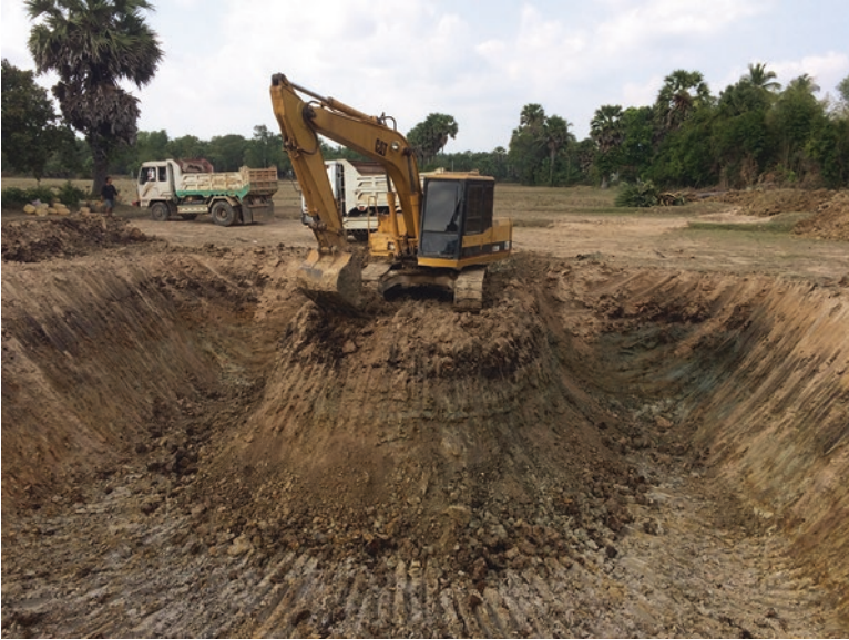
Photo 4.5 A local family hires an excavator to dig a private pond for small-scale irrigation
