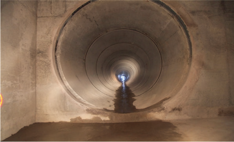
Fig. 3.7 A 3 m-diameter drainer and storage tank at the Wuluju Rainwater Pumping Station
