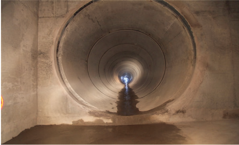
Fig. 3.7 A 3 m-diameter drainer and storage tank at the Wuluju Rainwater Pumping Station
