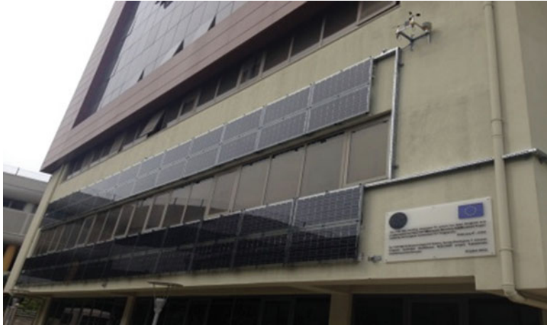
Fig. 63.1 A picture of the BIPV system installed [8]
