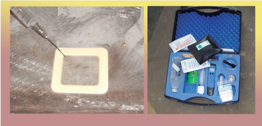
Fig. 4 Salt test in the surface to be painted
