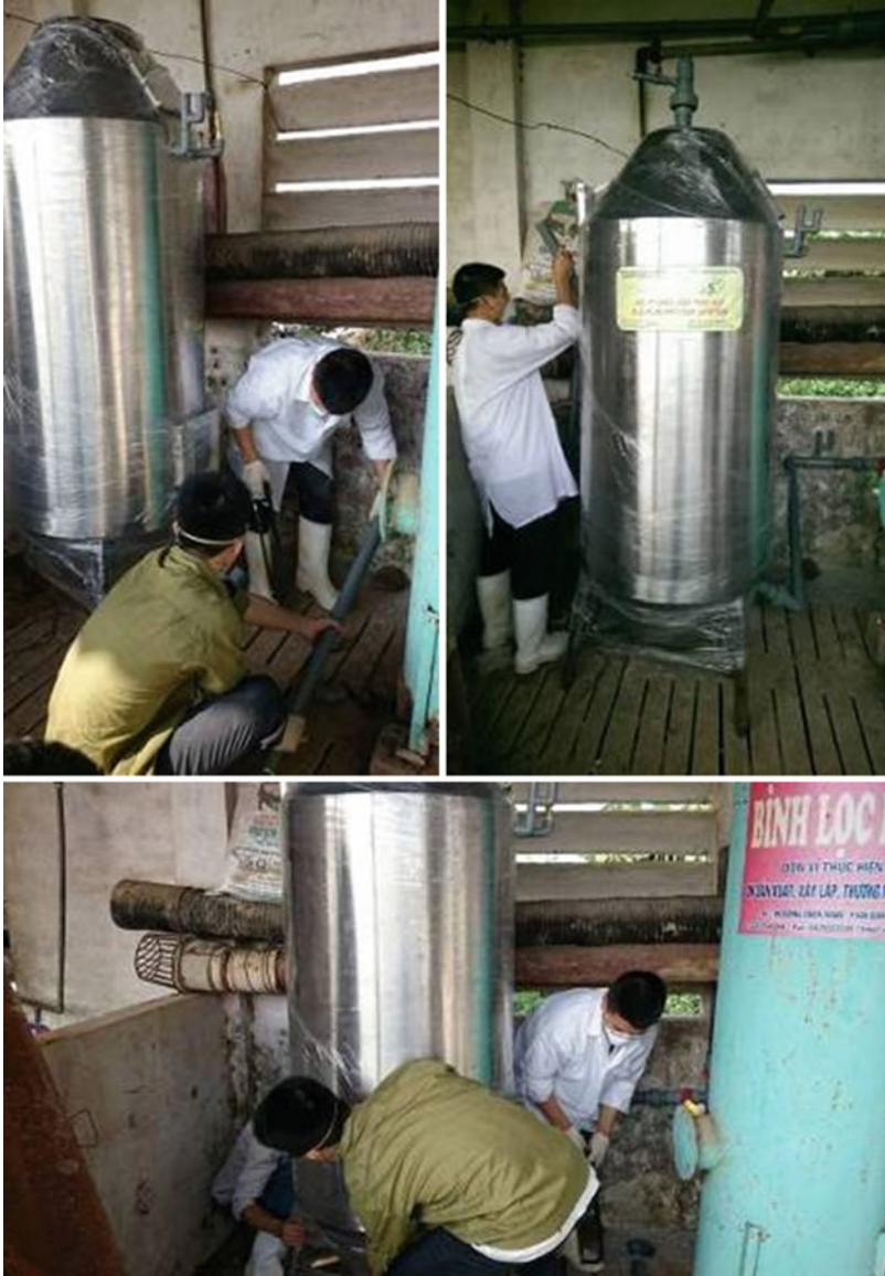
Picture 7 H 2 S adsorption system installed at the Thanh Hung pig farm
