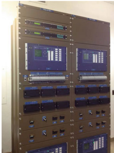
Typical PMU racks in a substation
