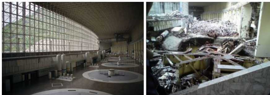
Fig. 10.2 Turbine hall of the Sayano–Shushenskaya power station before and after the accident in 2009 [2]
