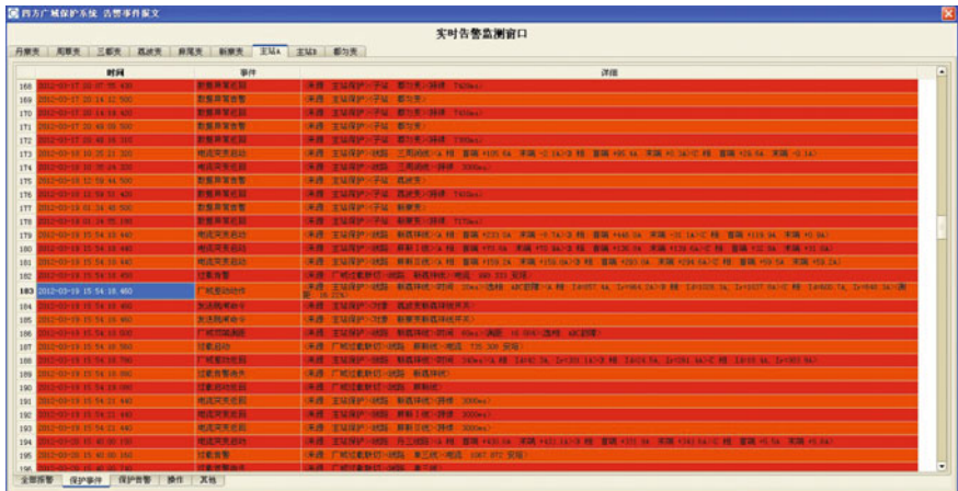
Fig. 5.23 Control commands displayed on the master station of WAP system
