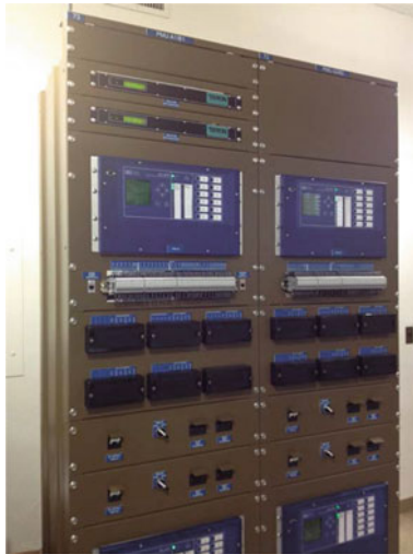
Typical PMU racks in a substation
