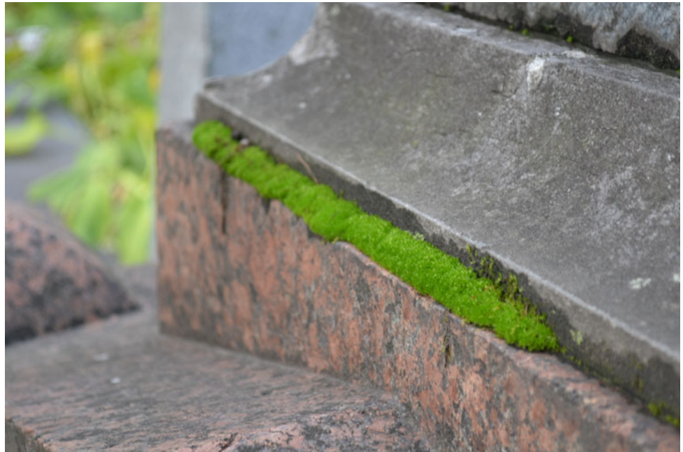
Fig. 3.24 Development of mosses along the junction of stone elements of the monument, where the substrate is more humid. Necropolis of the 18th century
