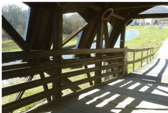
Fig. 1.21 Detail of arch bridge with wheelchair access over a tributary of the River Hron (Kováčovský potok) on hiking path in Zvolen, Slovakia ( Photo Jakubisová )
