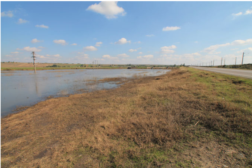
Fig. 6.13 Water accumulation behind the embankment and the failure of pumps (in the background) to eliminate excess water in time. Source Author
